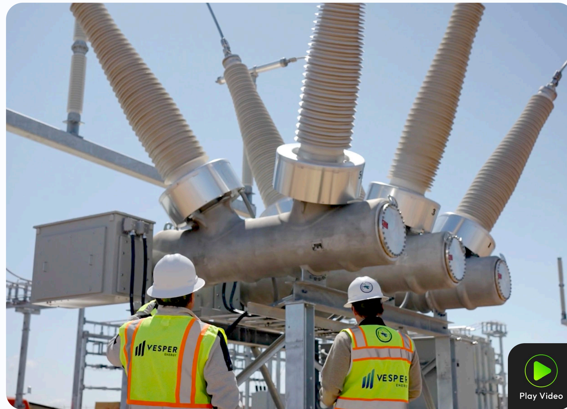
Pictured: Vesper employees at their solar site in Swisher County, Texas
